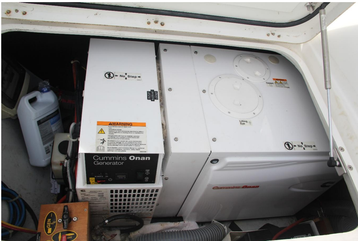
Cummins/Onan 13.5kW diesel generator
