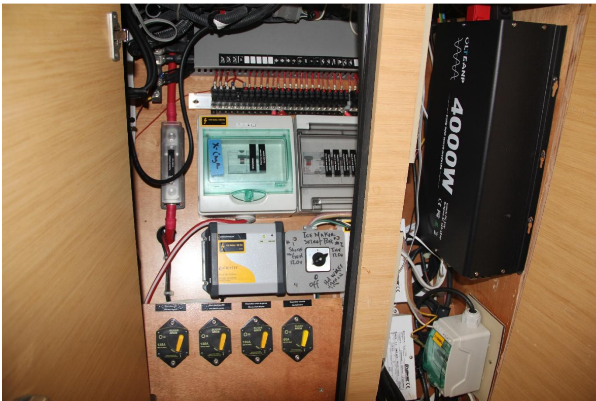
Integrated/isolated 4000W AC inverter/charging system; note labeled switches
